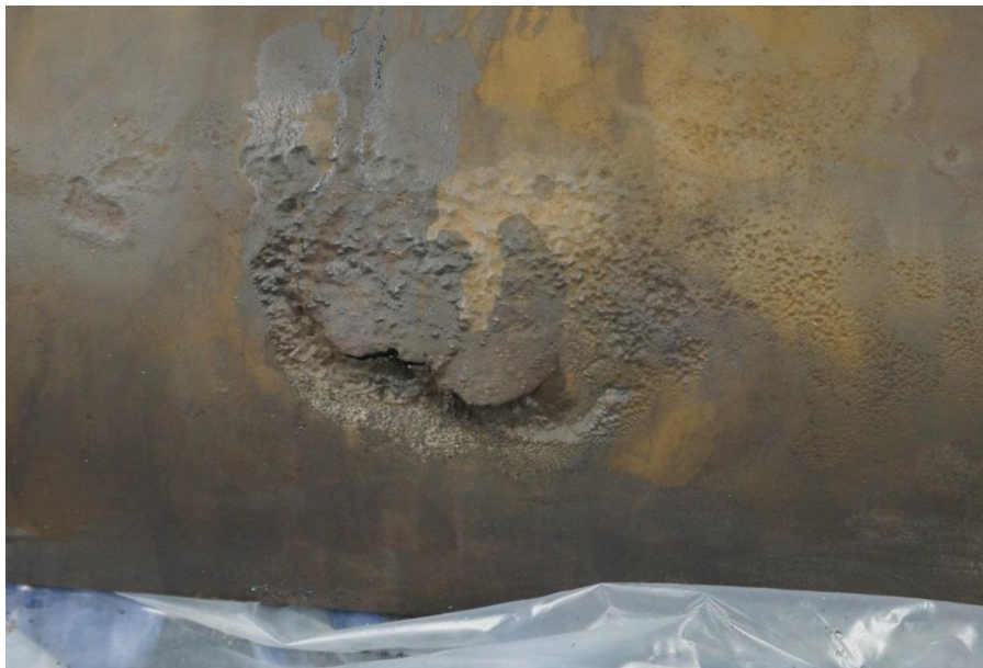
Figure 5. Pipe External Surface at the Line 901 failure site after cleaning.
